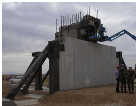
FIGURE 3 TYPICAL CONCRETE CLADDING WALL INSTALLED ADJACENT TO AIR BLAST/PROGRESSIVE COLLAPSE TEST ARTICLE.
