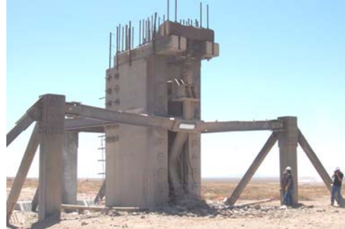
FIGURE 13 SIDEPLATE ® MOMENT CONNECTION: COMPLETE COLUMN DEMISE AND SEVERE GLOBAL DEFORMATION WITHOUT COMPROMISING THE CONNECTION, ABSENT FLOOR GRAVITY LOADS.
