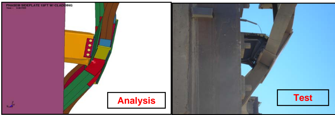
FIGURE 16 SIDEPLATE ® MOMENT CONNECTION: PREDICTIVE BLAST ANALYSIS CORROBORATES INELASTIC TWIST AND VERTICAL DISPLACEMENT OF DOUBLE-SPAN BEAM.
